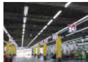
Service pits that use fluorescent lighting with higher energy efficiency
