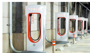
Tesla's Supercharger fast-charging stations installed at A PIT AUTOBACS KYOTO SHIJO
